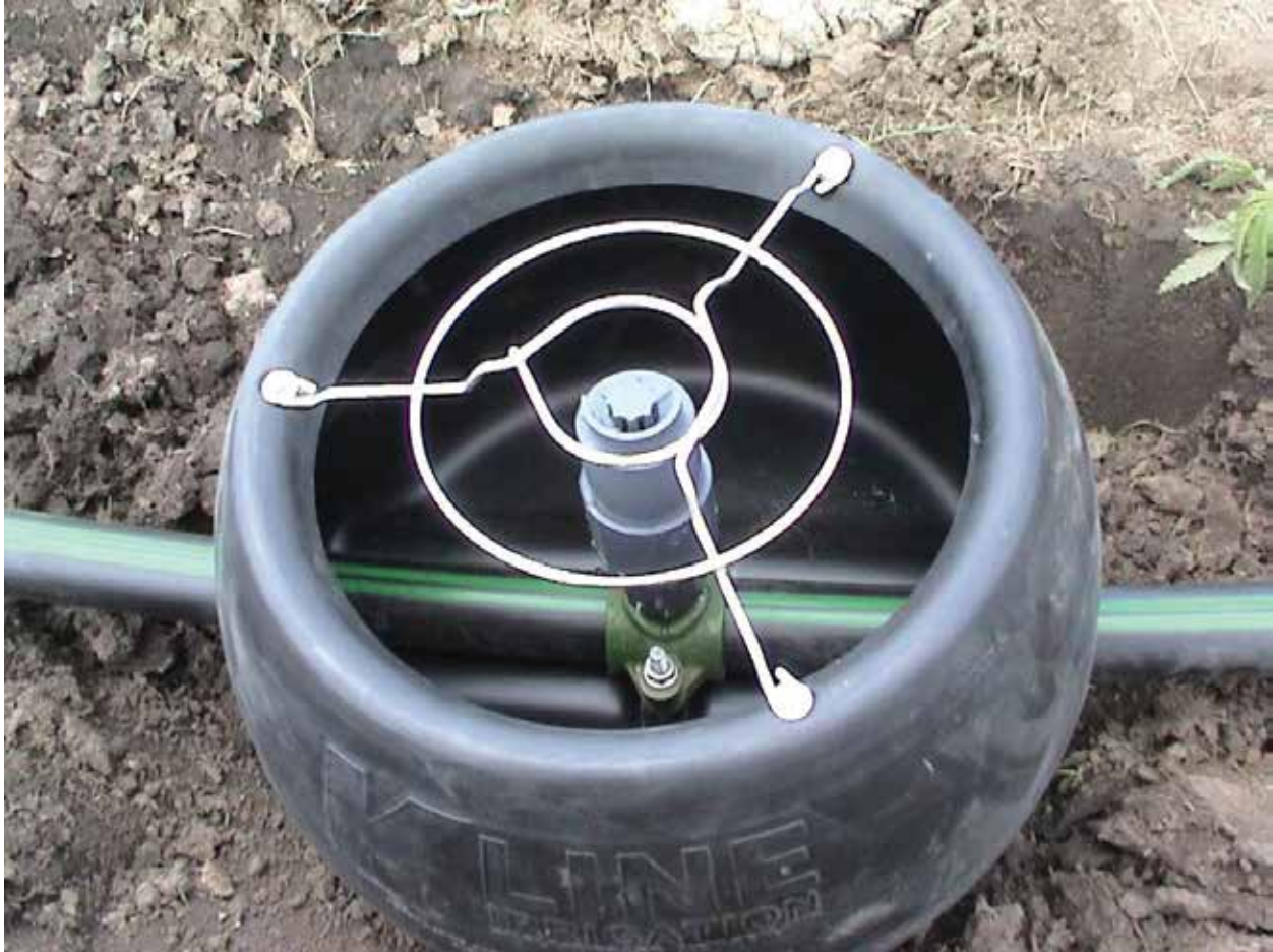
Figure 12. Close-up of portable air/vacuum vent within protective pod. Photo credit Jason Gross.
